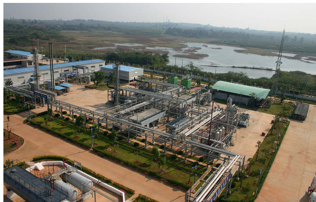
Small-scale LNG modular plants offer reduced commissioning time and costs
