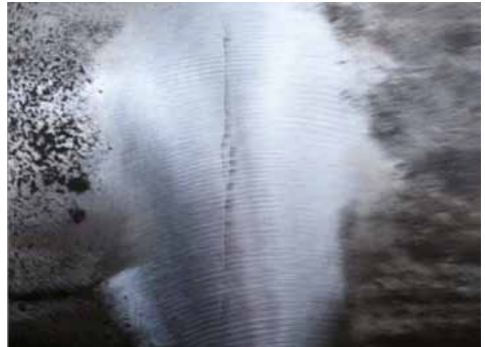
What appeared in MFL data to be metal loss, was in fact a circumferential crack coincident with a bending strain peak.
