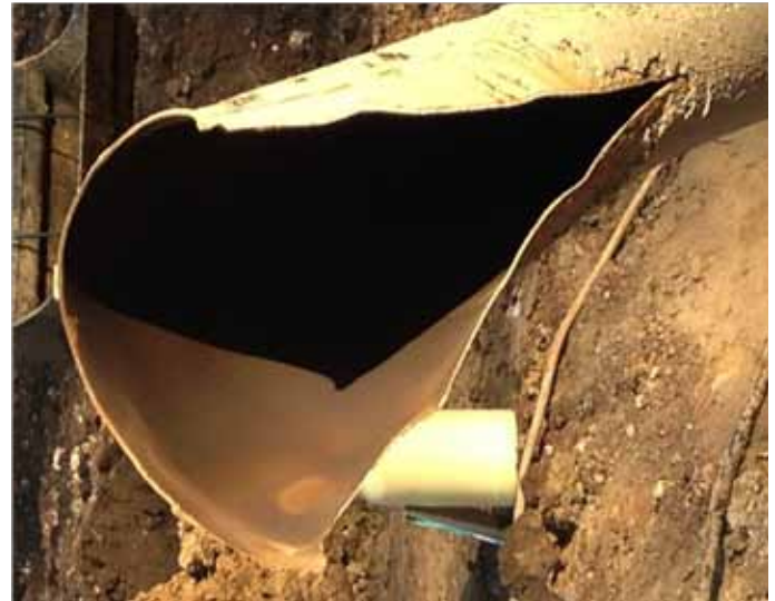
The pipe steel was in excellent condition; the rupture resulted solely from high shear forces caused by gradual land movement.
