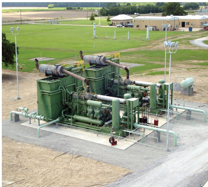
MH64 compressors in Rayne, Louisiana
