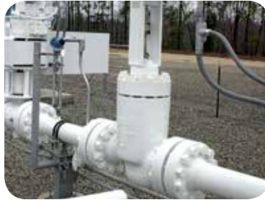
49000 Series with V-LOG* Trim in a Gas Storage Field
