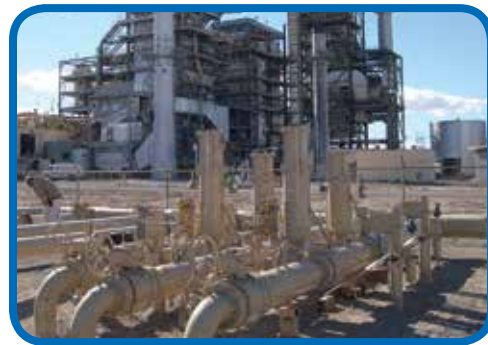
Figure 10 - Slam Shut and Fast-Acting Monitor Regulators Natural Gas Fired Power Plants (Power Generation Industry) Fast-acting monitor regulators and Slam Shut valves provide the ultimate protection to natural gas Fired turbines from overpressure occurrence. These monitor regulators and slam shut valves utilize Surge Design RPSR actuators to ensure quick stroking and minimize potential of damage to downstream pipe and equipment in the event of potential overpressurization. Slam Shut valves and fast stroking monitor regulators are standard to most Becker pressure regulators stations that feed power plants due to their reliability and purpose built design.
