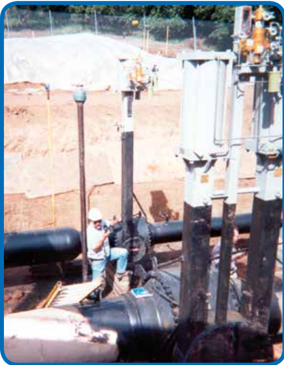
Figure 11 - Installation of Becker Below Ground Regulators (Prior to Backfill) A large natural gas transmission/distribution company based in Southern California installed Becker Below Ground Ball Valve Regulators to achieve maximum noise attenuation, minimal maintenance, and optimum cost effectiveness. The Below Ground Regulator can provide up to 37 dBA additional noise attenuation with minimal additional cost. Two different size Below Ground Ball Valve Regulators are shown here. 16" Bore Below Ground Regulators are shown in background, while 30" bore Below Ground Ball Valve Regulators are shown in foreground. The Below Ground Ball Valve Regulators are shown during installation, prior to backfill of the regulator station.
