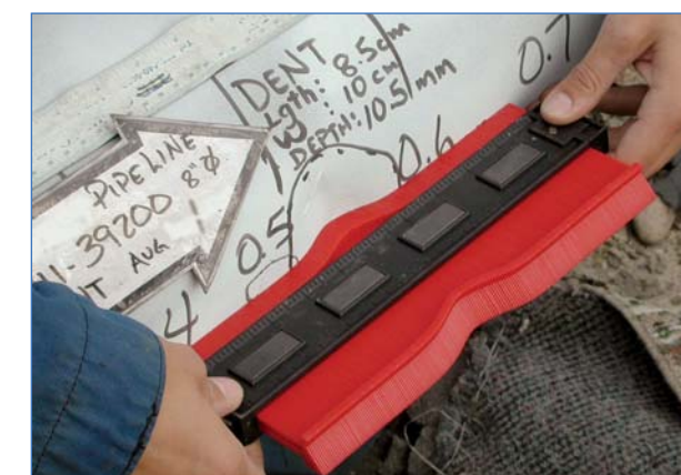
IMU provides GPS co-ordinates for location of identified defects to an accuracy of +/- 1.5 m.
