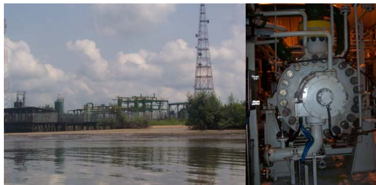
Figure 3: Pictures of Compression Plant (left), Installed HP Unit (right)
